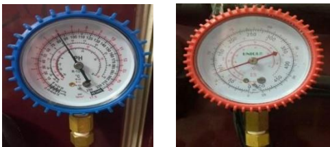
Figure: Suction and Discharge pressure gauges
