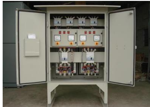
Plate 1: Electrical Feeder Pillar
