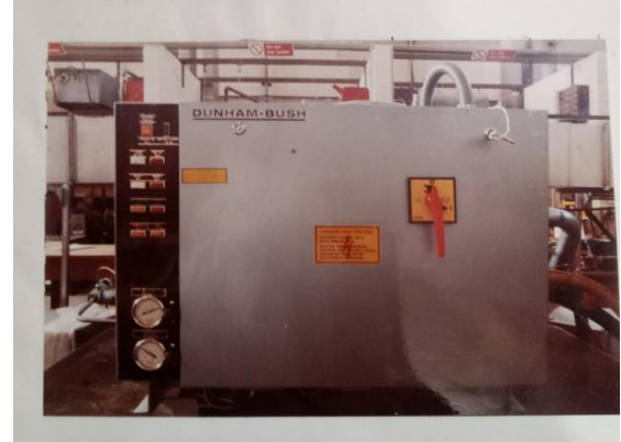
Plate 1: The Chiller that was investigated.
