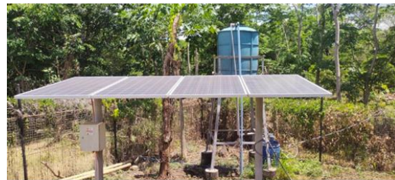
Picture 2. Solar-powered Irrigation System
