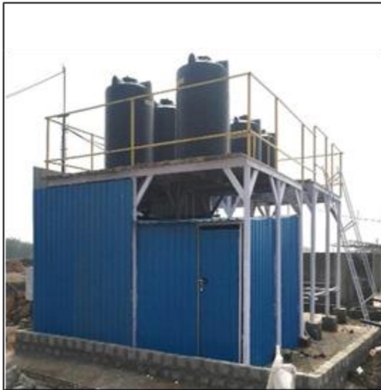
RO Plant at Workers Camp – As per standard practice
