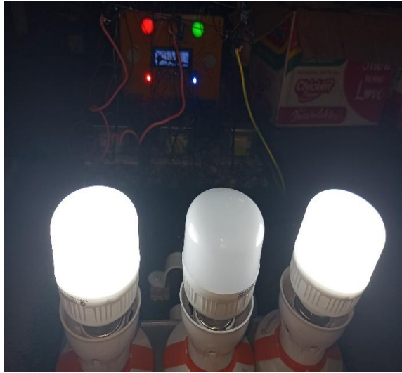
Figure IV-3 The tripped off yellow phase bulb
