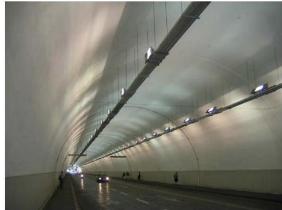
Figure 1. Real-World Validation: Nano- \text{TiO}_2 Coating for Tunnel Air Quality Management (adopted from [3])
