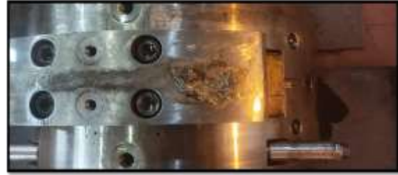
Figure 3: Electrical discharge markings at bearing torus support.
