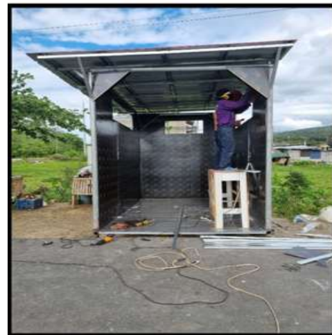
Fig. 2. Fabrication of the developed mobile study shelter with banana fiber roof insulation.
