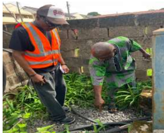
Fig. 7. Field engineers conducting insulation resistance measurements on the distribution network at ACU. The researcher (right, in orange safety vest) records readings while the technician manages test connections.
