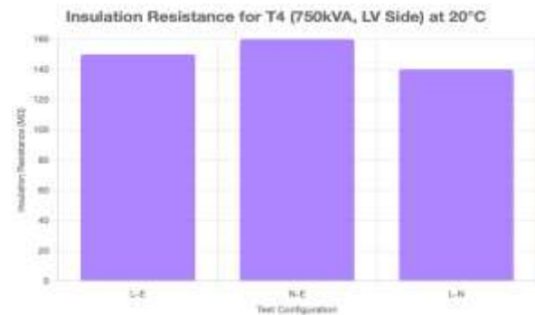
Fig. 12. IR test results for T4 (750 kVA, LV Side) at 20°C L-E: 150 MΩ, N-E: 160 MΩ, L-N: 140 MΩ. All values significantly exceed the IEEE standard (PASS).
