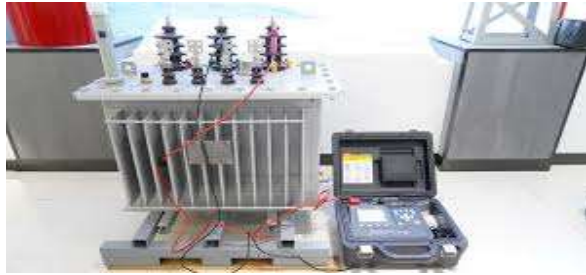
Fig. 4. Distribution transformer under test connected to the Megger MIT1025 insulation resistance tester.
