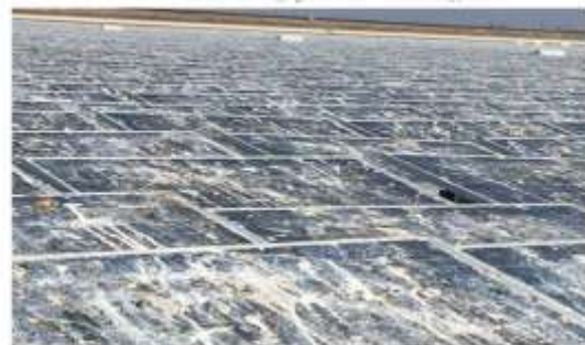
Figure 3: Bird Droppings on Solar Panel
