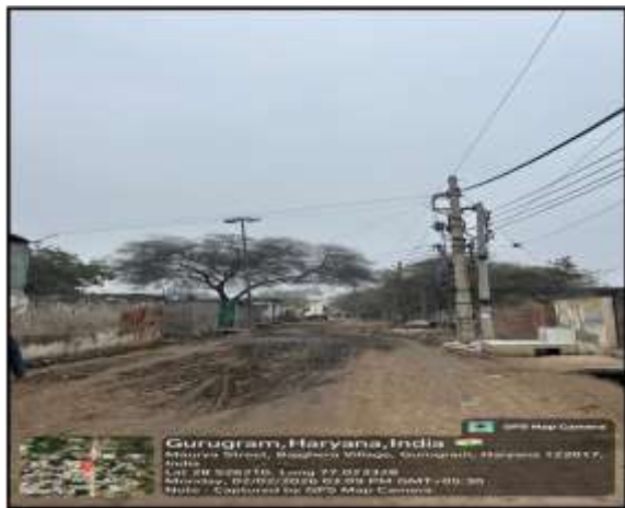
IMAGE 1:ON GROUND EVIDENCE OF POOR IMPLEMENTATION
