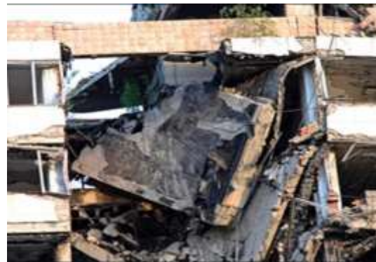
Fig. 1. Typical earthquake-induced damage to a building, illustrating the consequence of inadequate lateral-load resistance.
