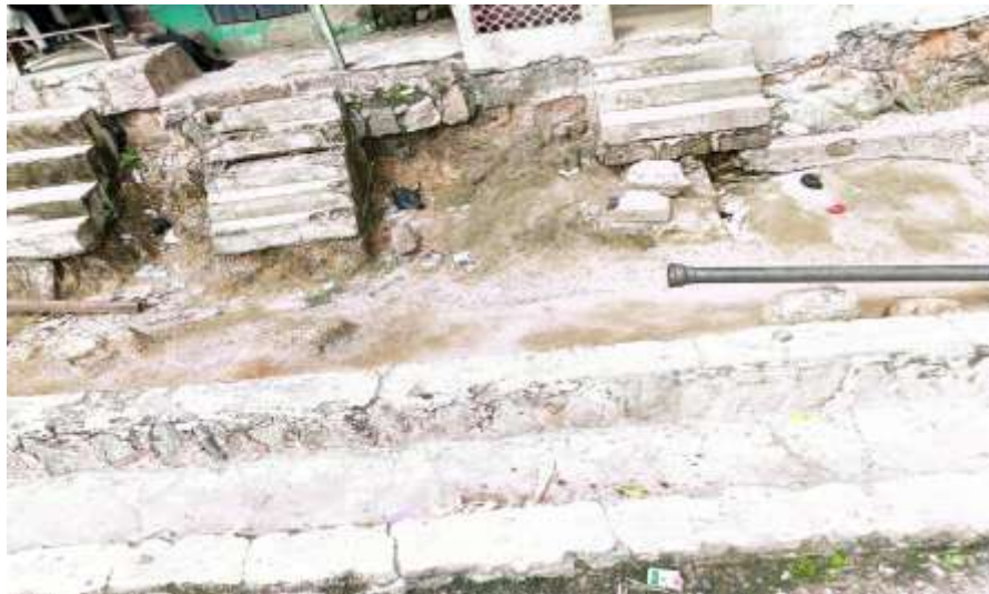
Plate 2: Water Service Pipe Exposed to Erosion, Corrosion, and Damage
