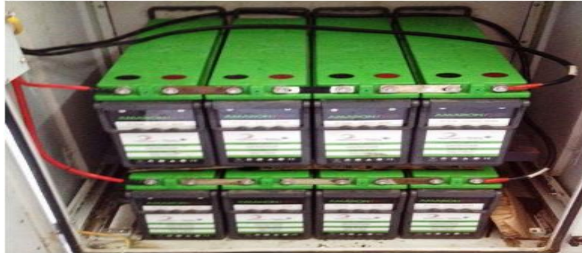
Plate 2 Battery Strings (Power/DC Storage Systems)
